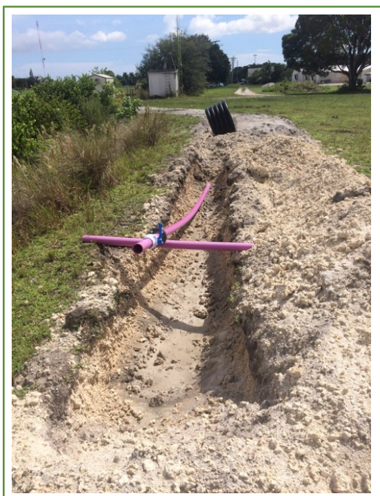
Picture 1. Four inches main line purple pipe brought to FLREC from Town of Davie Water Treatment and Water Reclamation Facility that is going to feed the research plots
